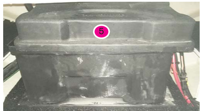
SEAKEEPER HOUSE BATTERY-UNDER MOTOR WELL
