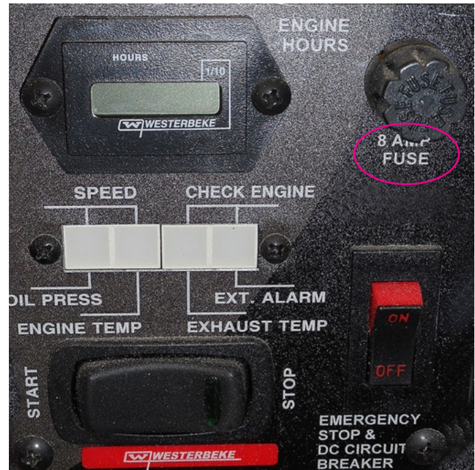
REMOTE GENERATOR PANEL SHOWING TOGGLE STYLE START/STOP SWITCH AND EMERGENCY STOP AND DC BREAKER
