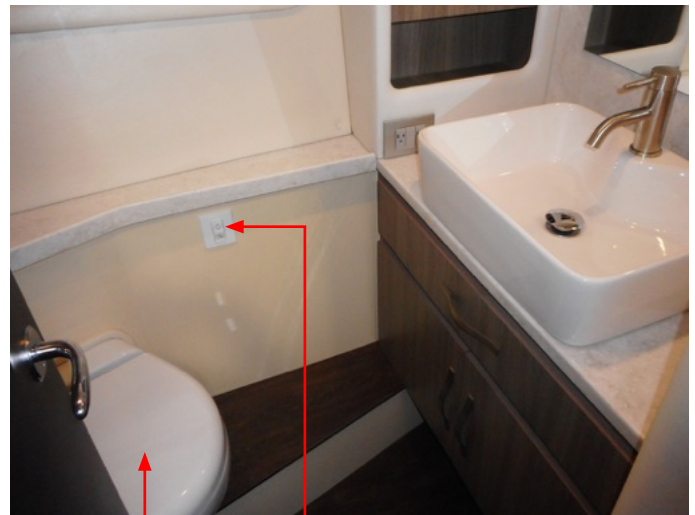
VACUUM STYLE TOILET
